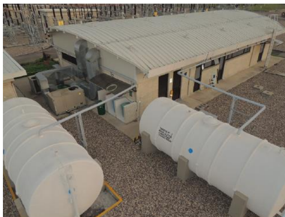
Figure 1. Rainwater Collection System at ISA ENERGÍA COLOMBIA
